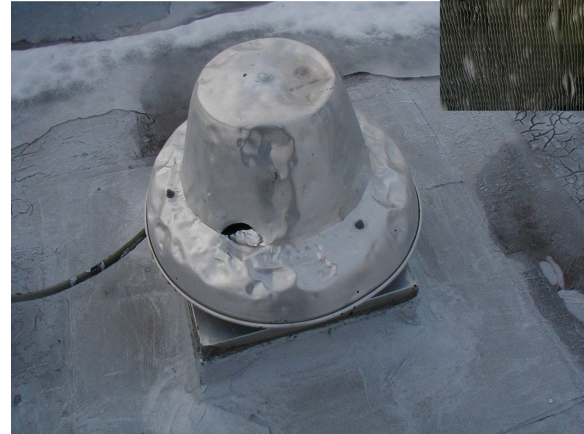
Photo 2, Hail Damage, Roof Exhauster
