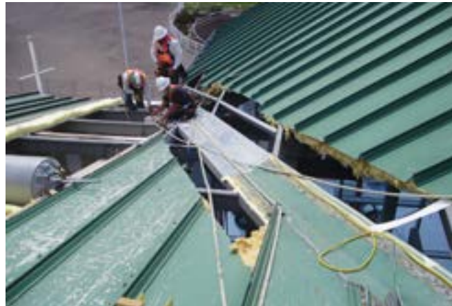
Removing and replacing the standing seam panels on a roof with an open frame. PHOTO COURTESY OF MCELROY METAL
