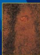
Galvanized test panel covered in red rust after 18 years in rural environment.
