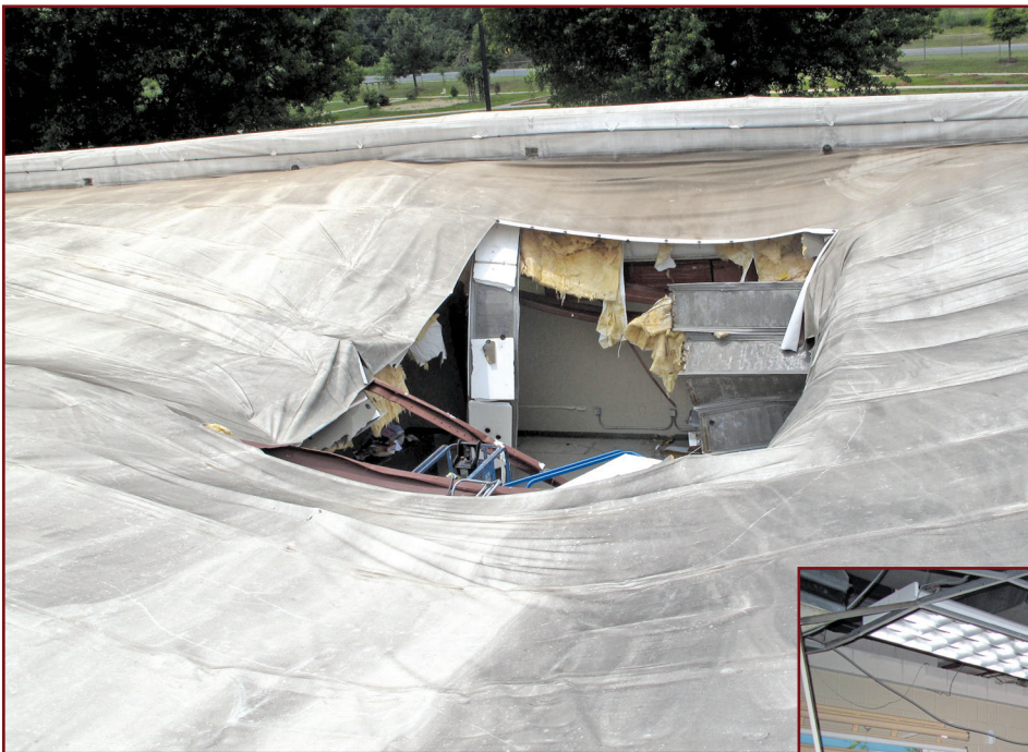
Figure 2 – This same building roof collapsed due to several factors related to a single-ply re-cover.
