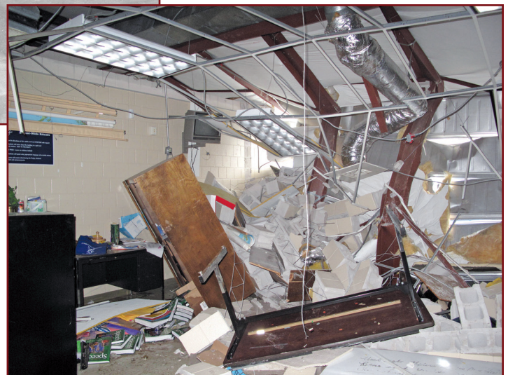
Figure 3 – Interior shot of collapse.
